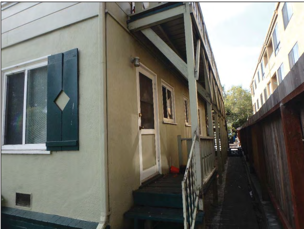
Figure 5. Detail of First Story of Entry Point On Northwest Elevation (View to South) IMG#: P9060007
