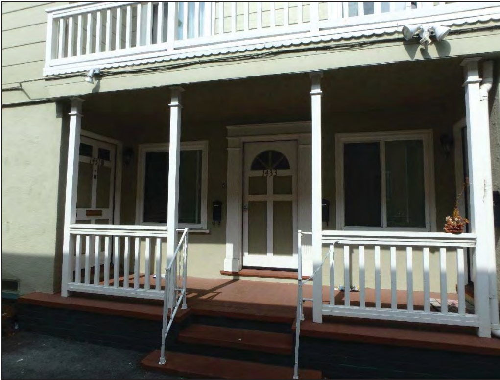
Figure 2. Detail of First Story of Entry Point on Southeast Elevation (View to Northwest) IMG#: P9060009
