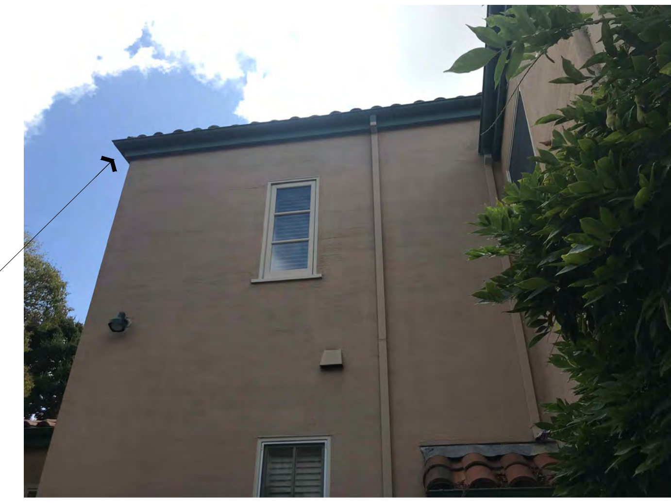
EXISTING ROOF PROJECTION 1-HOUR FIRE RESISTANCE-RATED CONSTRUCTION PER 2019 CRC R 302.1 OR 2019 CBC 705.2
