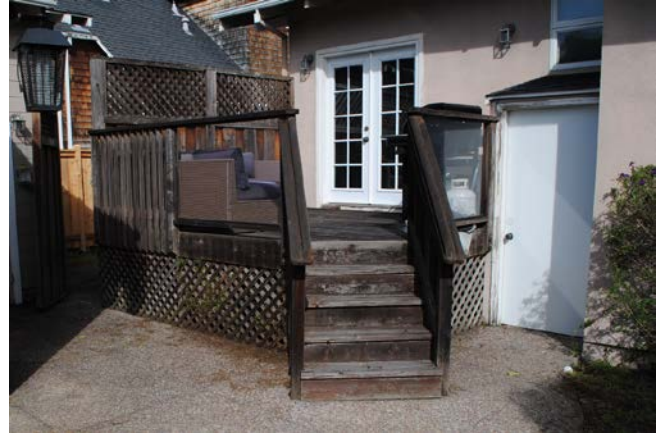
Figure 11. Wood deck at the west end of the rear façade, looking northwest.
