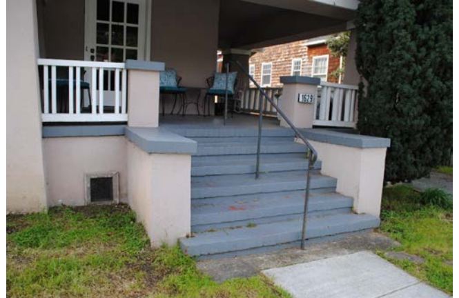
Figure 3. Detail of stairway leading to the entry porch on the primary façade, looking southwest.
