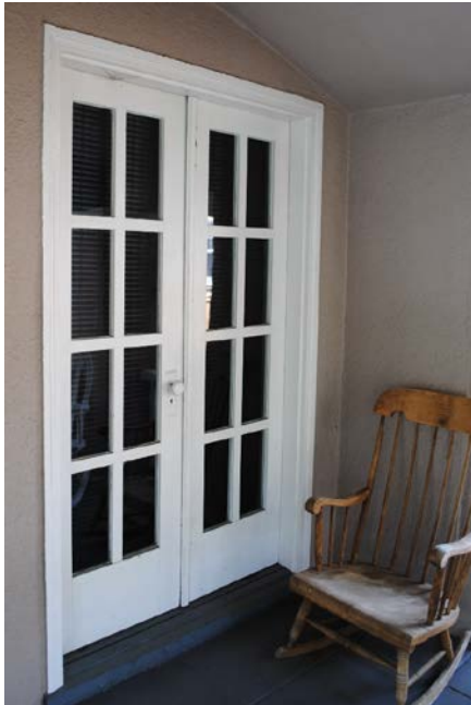
Figure 8. Glazed double-doors located on the west façade, leading to the entry porch.
