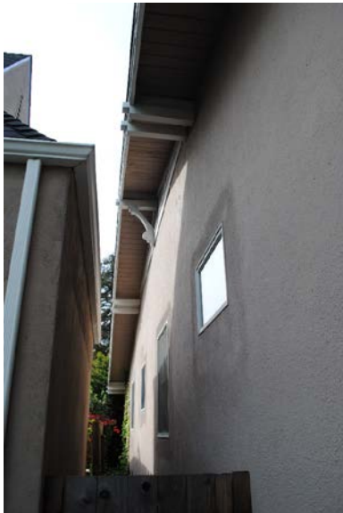
Figure 12. Partial view of east façade, looking south. Subject residence is on the right, and the neighboring home at 1625 Howard Avenue is on the left.
