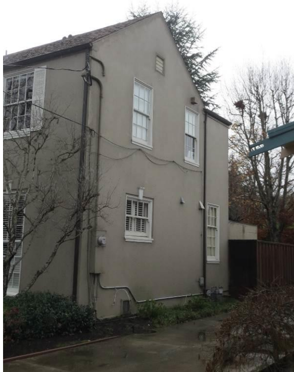
Figure 9. North façade and roof line, with primary façade partially visible at left, looking southwest from Cypress Avenue. Page & Turnbull, December 2014.
