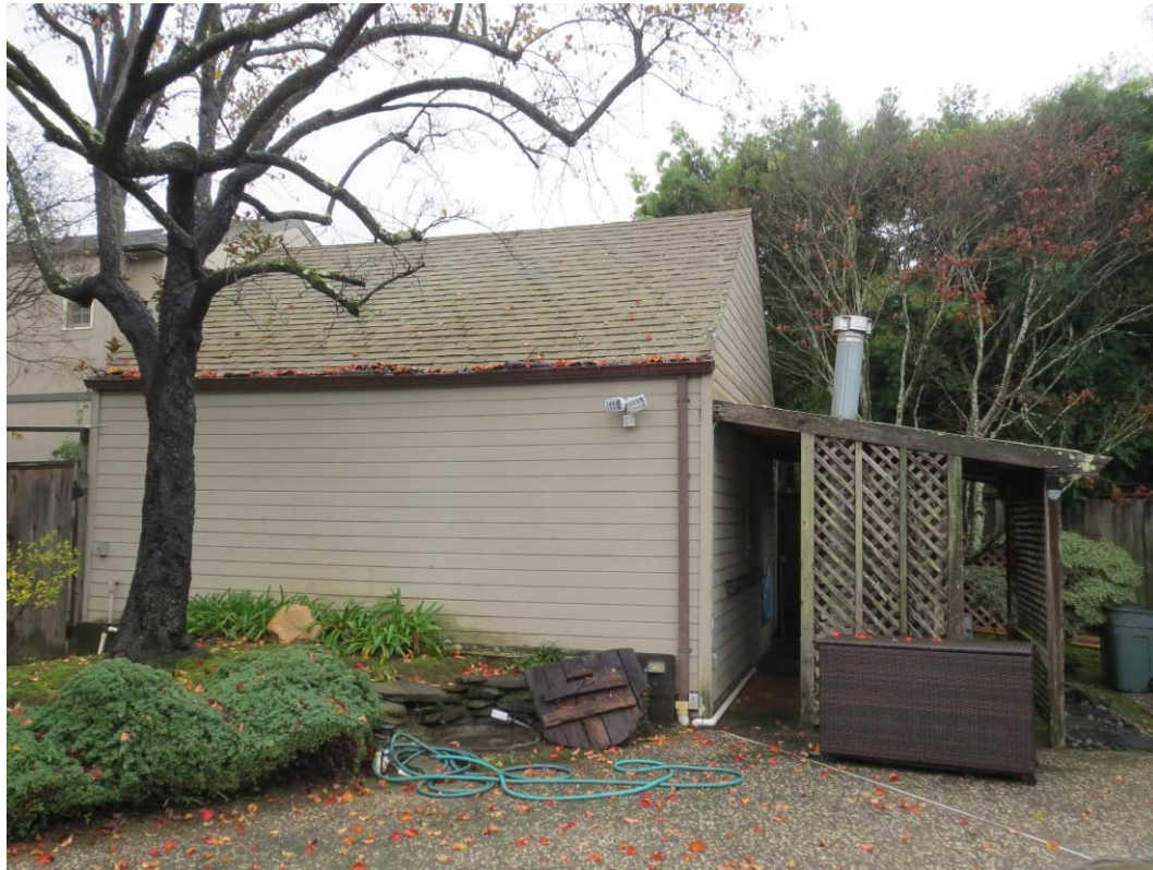
Figure 11. Garage, north façade showing lean-to at rear, looking south from rear yard. Page & Turnbull, December 2014.
