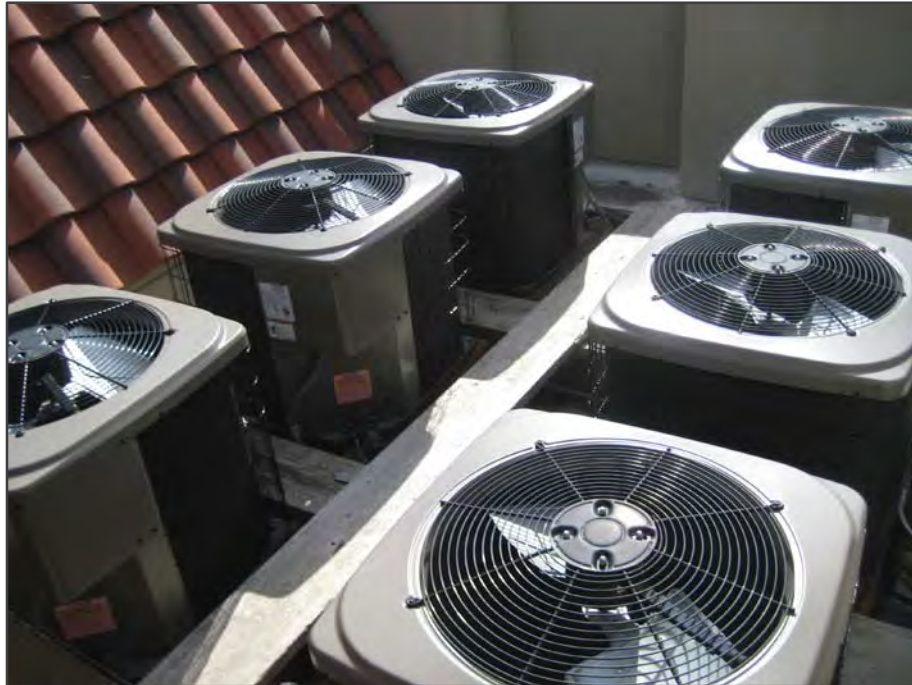
Photograph 1: Nine HVAC units on top of roof; located towards the front end of 1226 El Camino Real.
