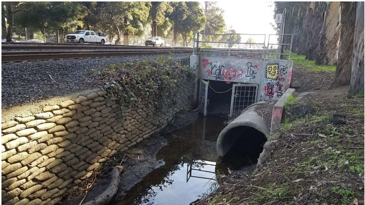
Photo 2. Burlingame Creek, looking upstream towards train station and confluence of two upstream storm drains that feed Burlingame Creek.
